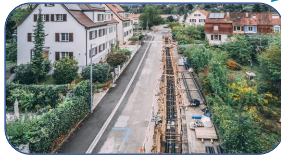
Riehen district heating network ©2018 Simon Havlik, Basel
