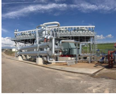
Soutz geothermal power plant
